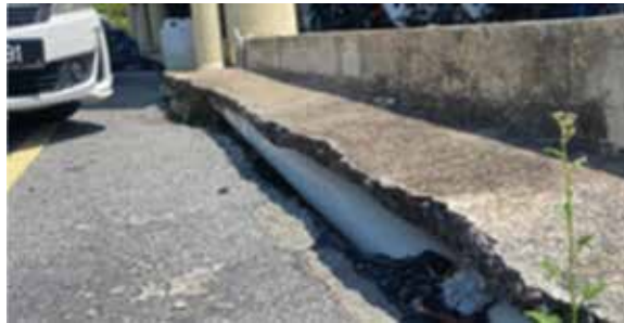
Kerosakan rainwater down pipe
